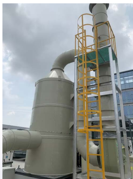
Acid Gas Post-Treatment System
