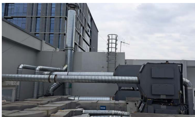
Activated Carbon Post-Treatment System
